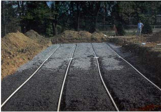
Figure 7. This is a view of a soil absorption system under construction. The pipes will be buried then covered by vegetation.
